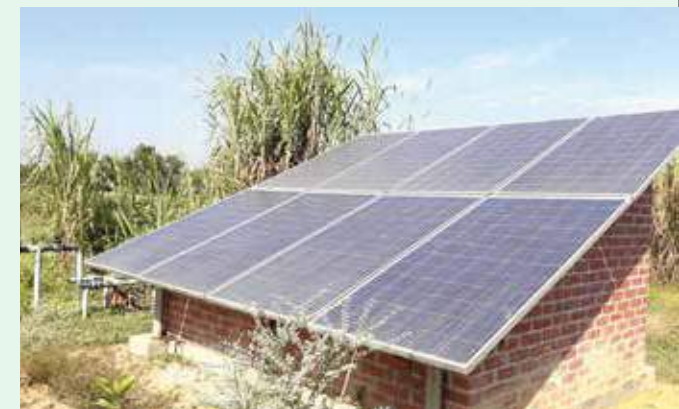
Solar irrigation pump
