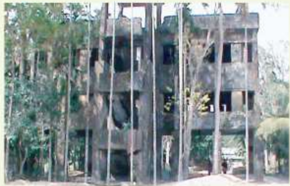
Condition of Cyclone Shelter to be Improved through Coastal Climate Resilient Project
