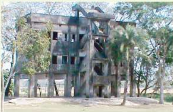
Condition of Cyclone Shelter to be Improved through Coastal Climate Resilient Project
